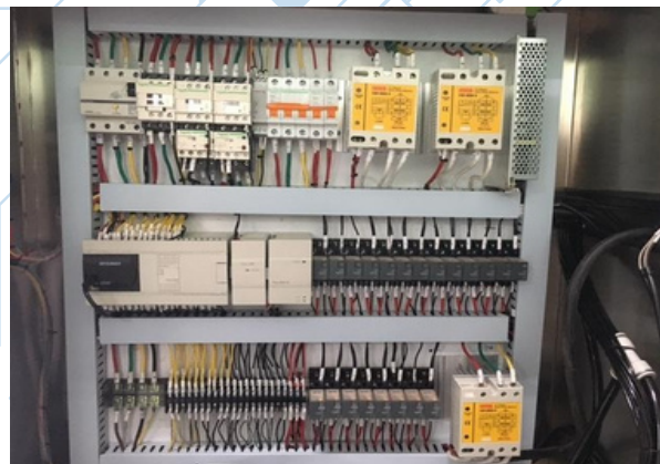
Electric control box
